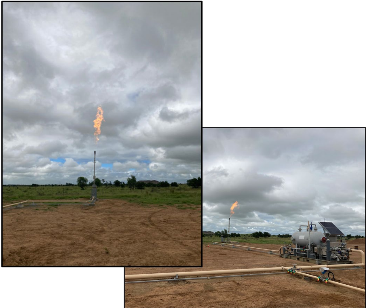
Figure 1: Sapphire 6 flare stack with blow down gas flaring during surface facility commissioning
